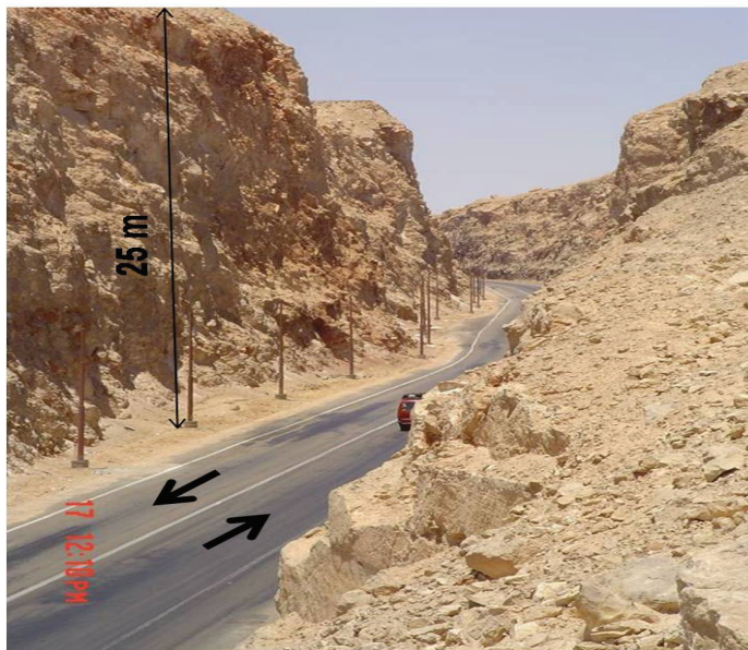
Fig. 2. An overview of the desert highway along the cut section showing the horizontal and vertical curvature of the road. The road has small shoulder, with no ditch, and one traffic lane in each direction.
